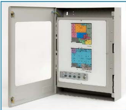
View showing mimic mounted on inner door
